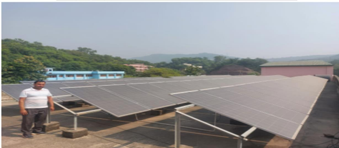
Roof Top Solar Grid: A Roof Top Solar Grid of 35 KW capacity with two way meter system has been fitted on the roof of arts block.
